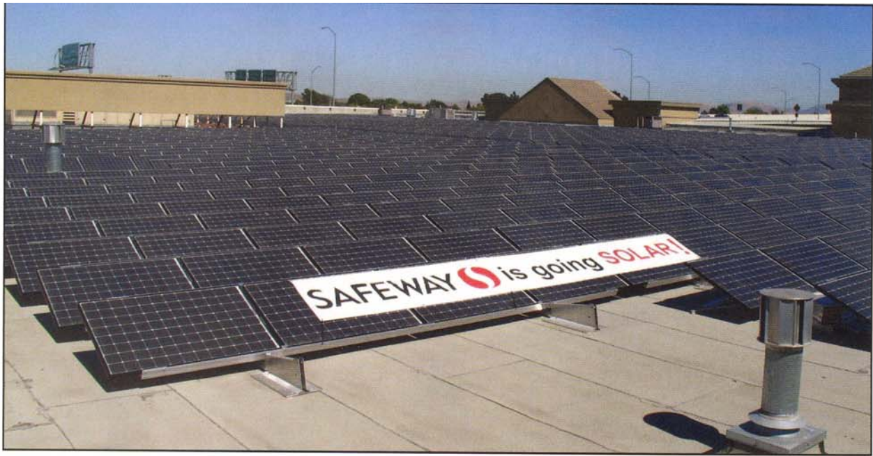
Nine Safeway stores, such as this one in Dublin, Calif., have more than 1,000 solar photovoltaic panels on their roofs, capable of providing 20% of the store's power usage. (Photo courtesy of Safeway.)
