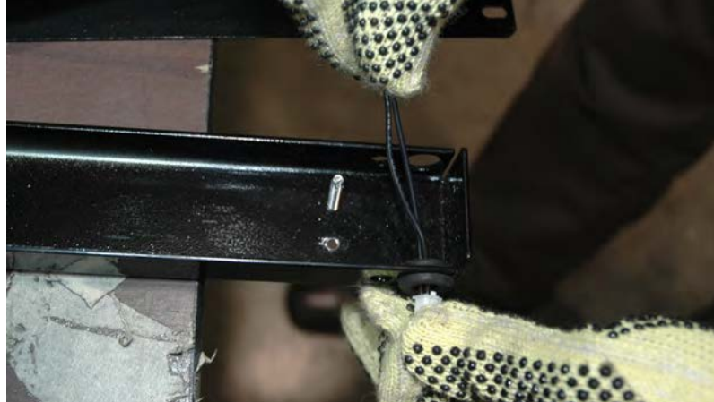
Heater wire pulled out of Bushing
