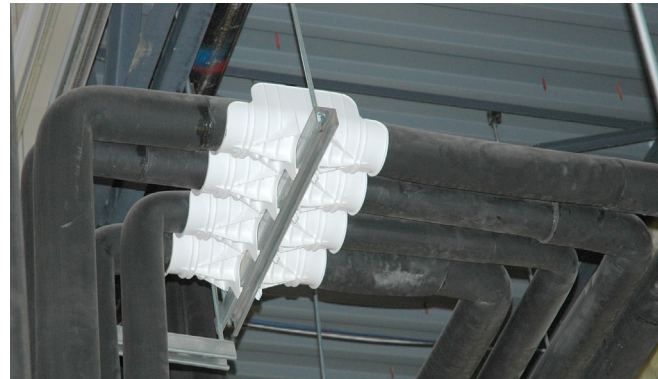
Ceiling Run with Supports
