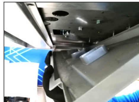
Condensate Pan Removed
