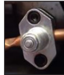
refrigeration line tapping valve
