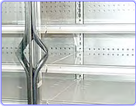
Improperly installed or damaged gasket
