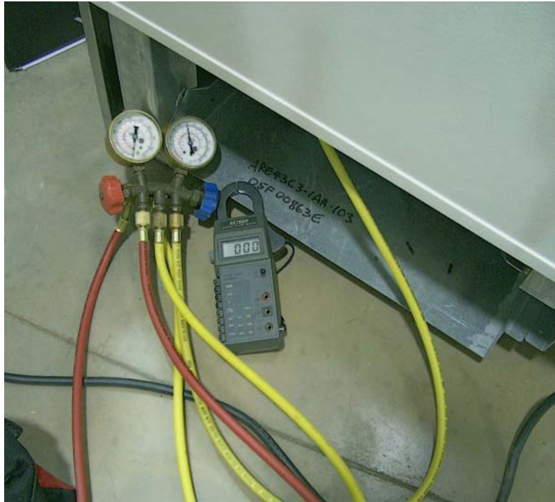
The CPR Valve is Located at the Left Upper Rear of the Compressor Compartment
