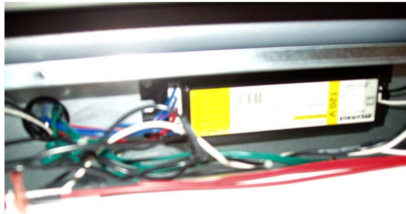
Figure 5 — Remove Shelf Lamp Ballast
