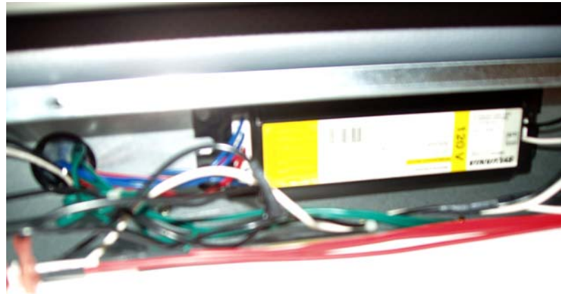
Figure 3 — Remove Shelf Lamp Ballast
