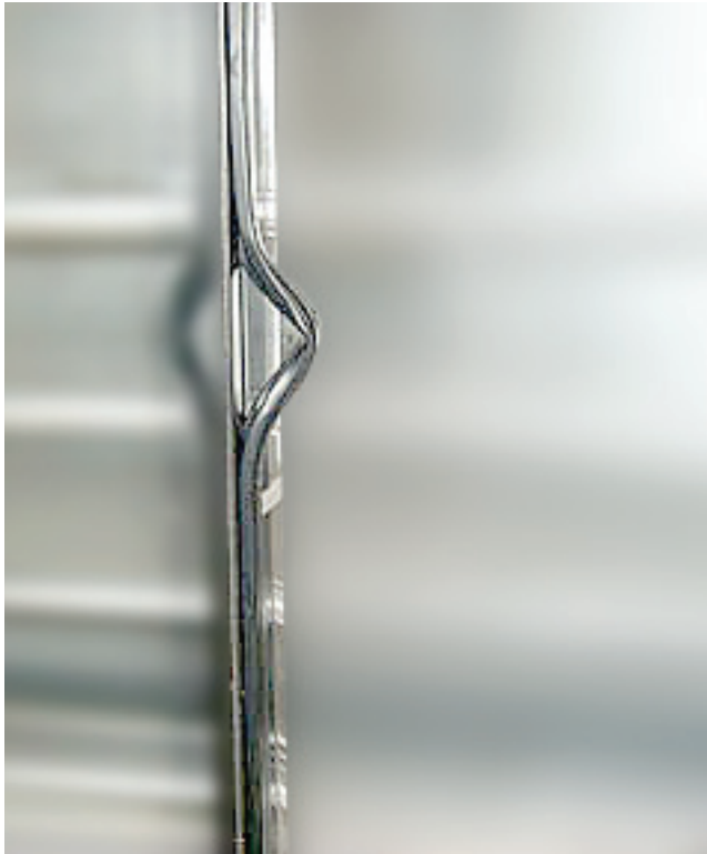
Improperly Installed or Damaged Gasket
